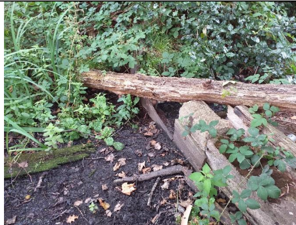
Fig 7: Debris and broken concrete on the spillway
